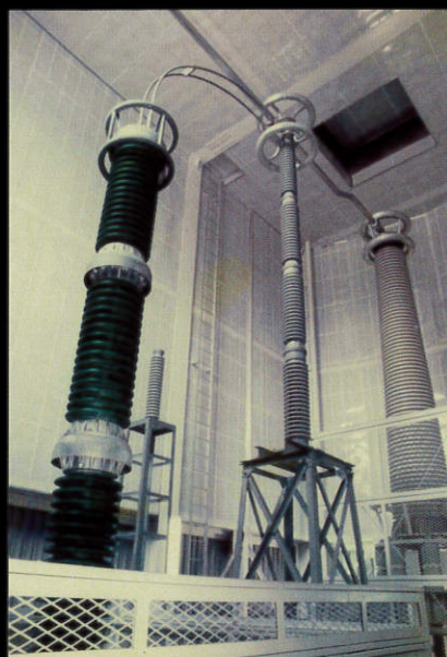
250kV surge arrester for protection of a DC transmission cable head for Hokkaido-Honshu HVDC Link
