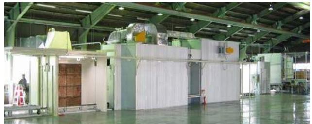
Continuous painting and drying furnace
