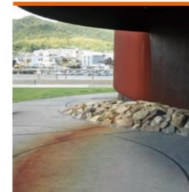
Discoloration due to rust in the shape of a flow or stream
