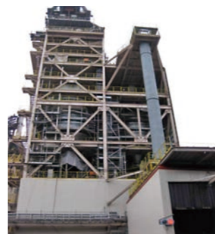
Pulverized fine coal injection equipment (with a zinc-rich primer)
