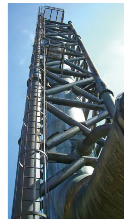
A smoke stack at a generation plant
